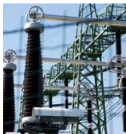
Electrical generation, transmission, distribution, installation & maintenance
