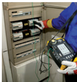
Tertiary and industrial maintenance, diagnostics & testing
